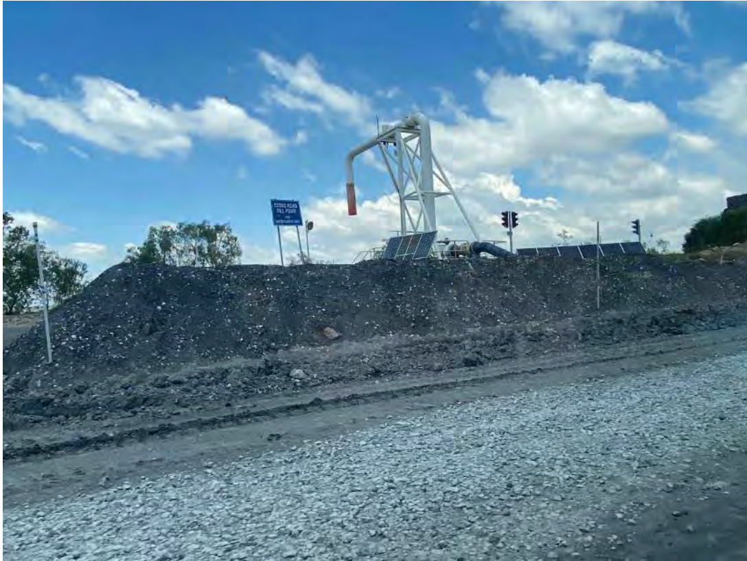
Plate 15 – Water truck fill point
