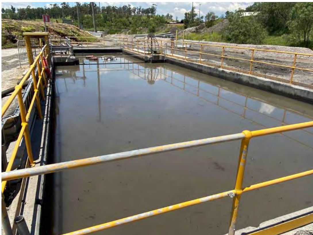
Plate 20 – Northern workshop oily water separator
