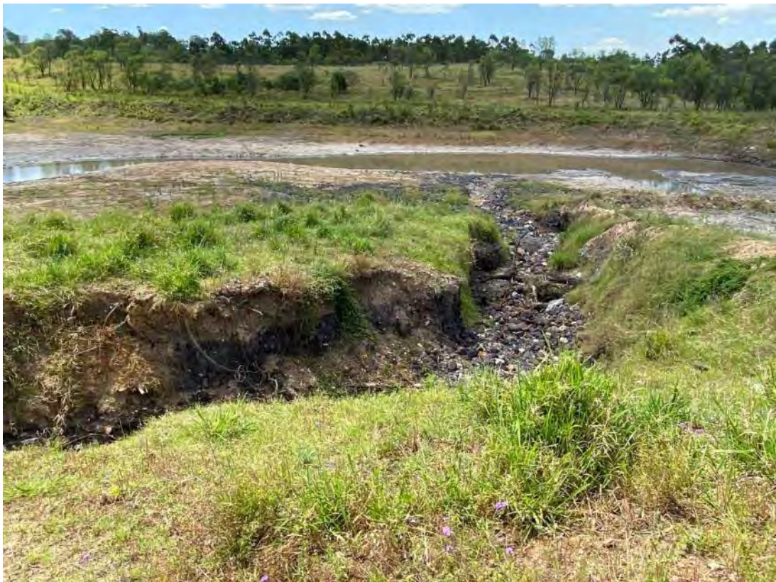
Plate 44 – Dam 5N outlet erosion
