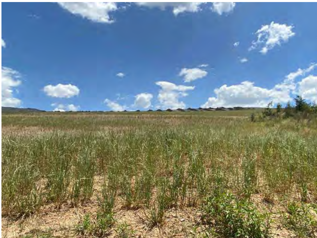
Plate 40 – Contour banks and drop structures within the inspected areas of the rehabilitation appeared stable and well-constructed.
