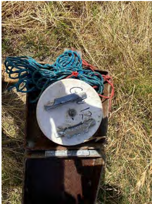
Plate 52 – Groundwater monitoring point cap adequately installed
