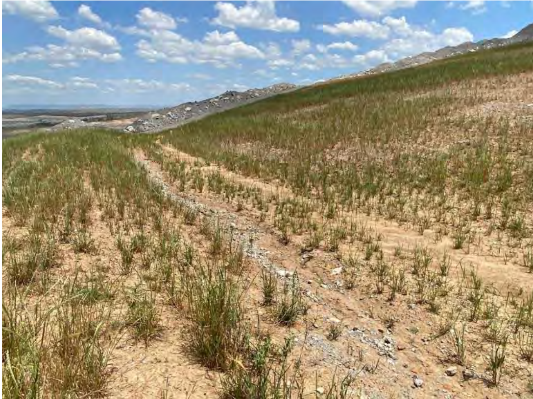
Plate 41 – Contour banks and drop structures within the inspected areas of the rehabilitation appeared stable and well-constructed.
