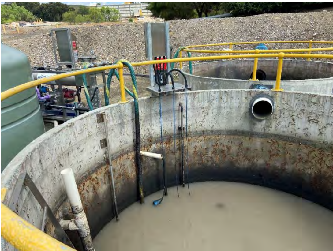
Plate 6 – Oily water separator in Southern Workshop
