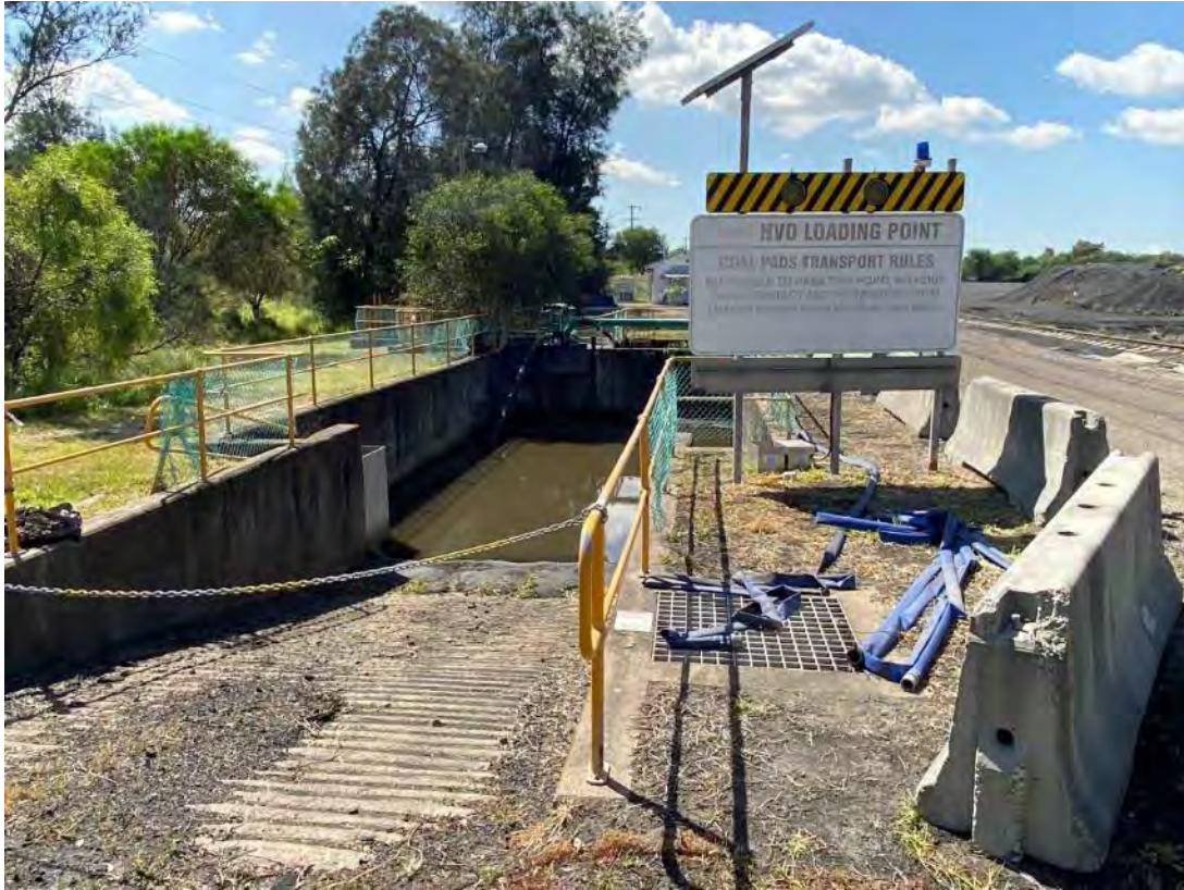
Plate 27 – HVO Loading Point Pollution Control Sump
