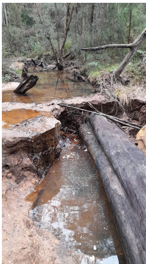
Figure 6.1. Erosion gully preventing access to the rear of the Condon View BA.
